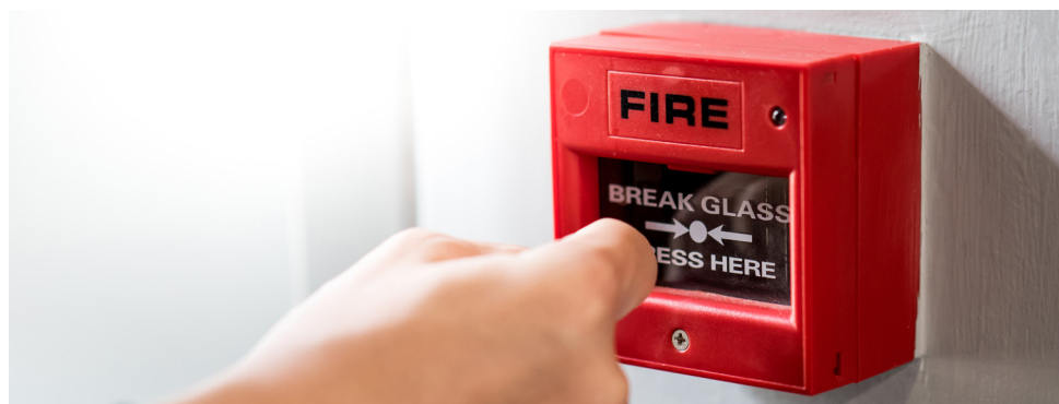
FIGURE 10–9 When a fire occurs, the fire alarm should be activated as quickly as possible.
